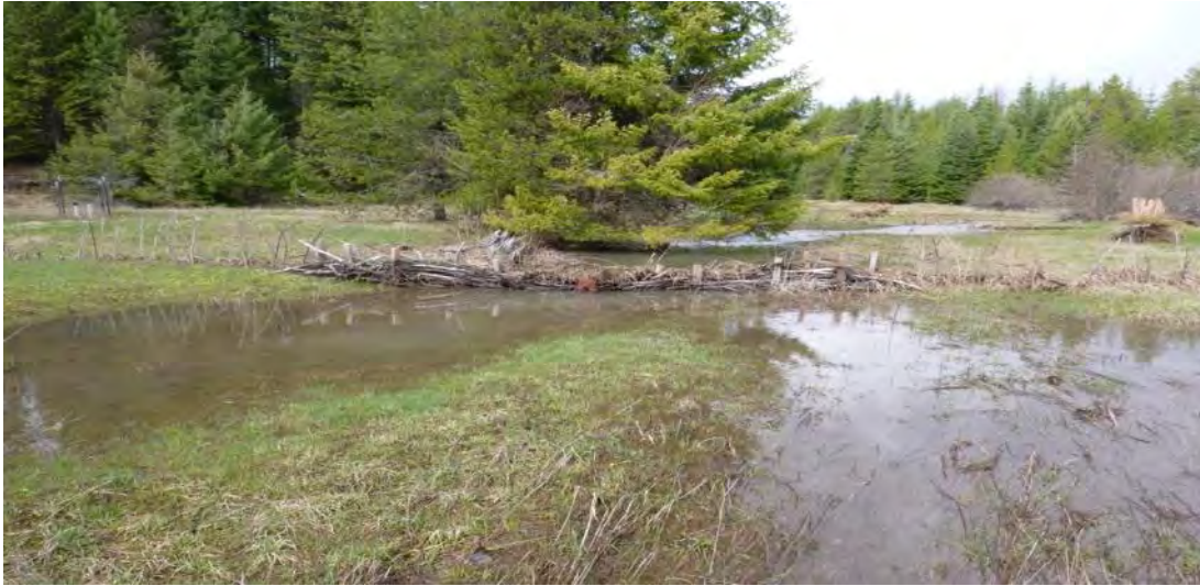
Figure 58. BDAs constructed with posts driven into the streambed woven with wicker weaves after peak flow.
