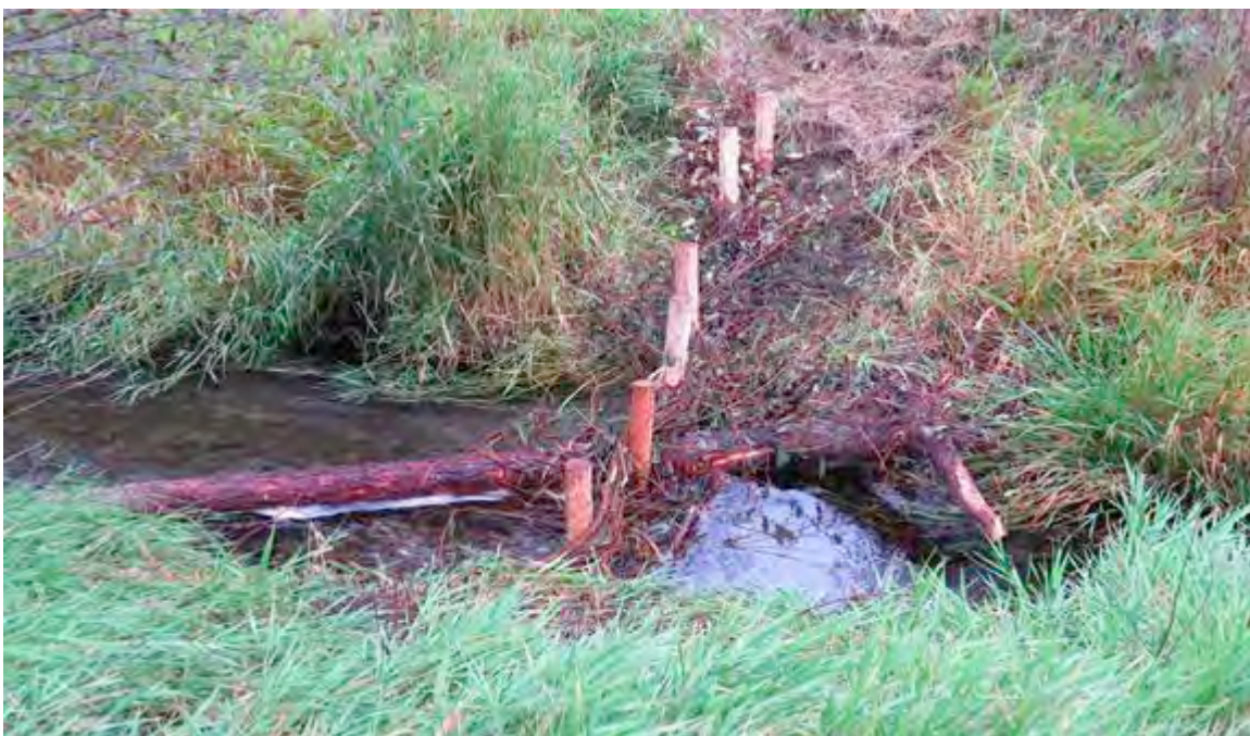
Figure 78: BDA – Two pilings extending onto the bank with LWD placed through the structure
