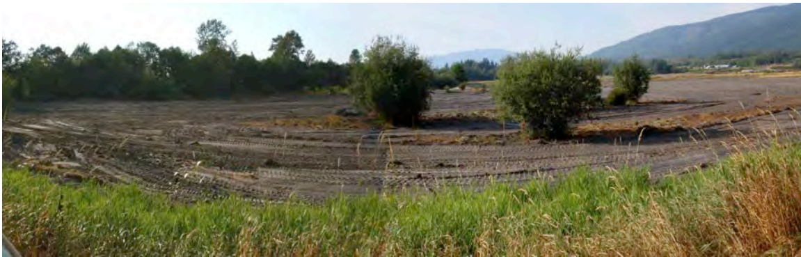
Figure 85: Photo of the restoration site during construction after removal of invasive reed canarygrass
