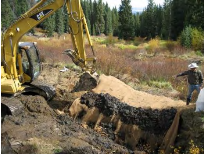
Figure 67: Breached dams were “plugged” with soil lifts wrapped in coir fabric and sod interwoven with live willow stems
