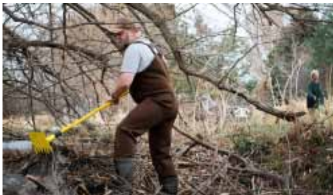
Chris Bachman of the Lands Council installed a pipe and cage system on Linda Jovanovich's land.
