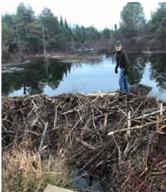
Tim Behrendt stands on the dam at Shawangunk Preserve near a new pipe and cage flow device.
