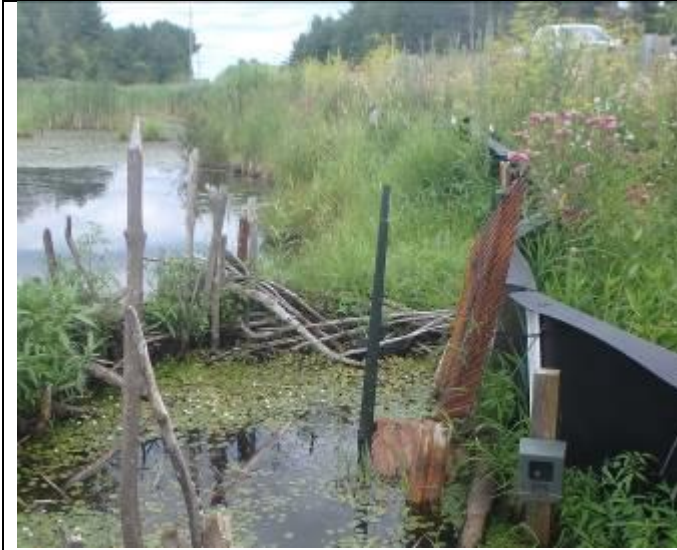
Photo 25: Stick debris on east side of diversionary dam on 10-Jul-16.
