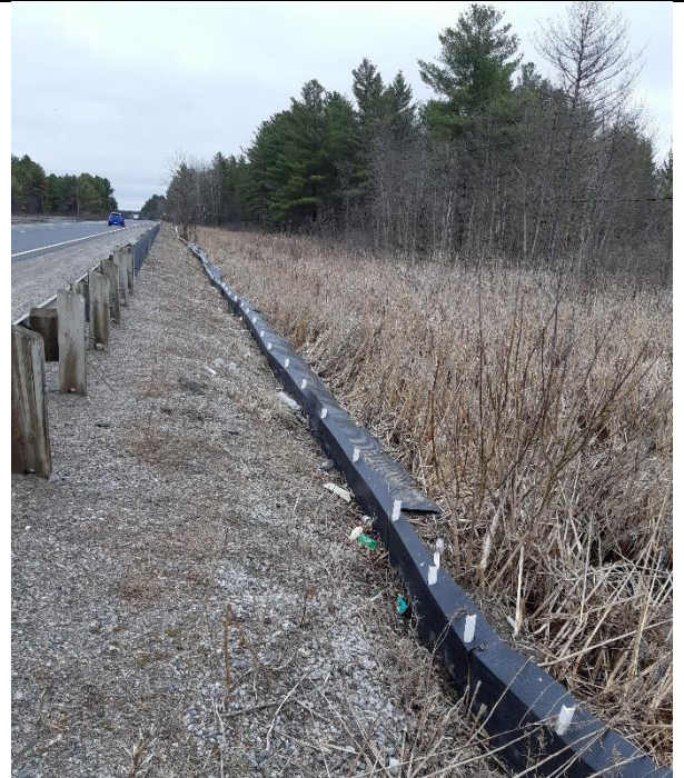
Photo 50: Viewing exclusion fence from top showing an approximate 30 cm below-grade installation (26-April-2019).
