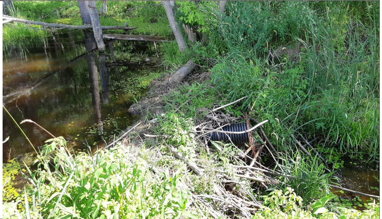
Photo 40: No water flow from pipe on July 4 th , 2019.
