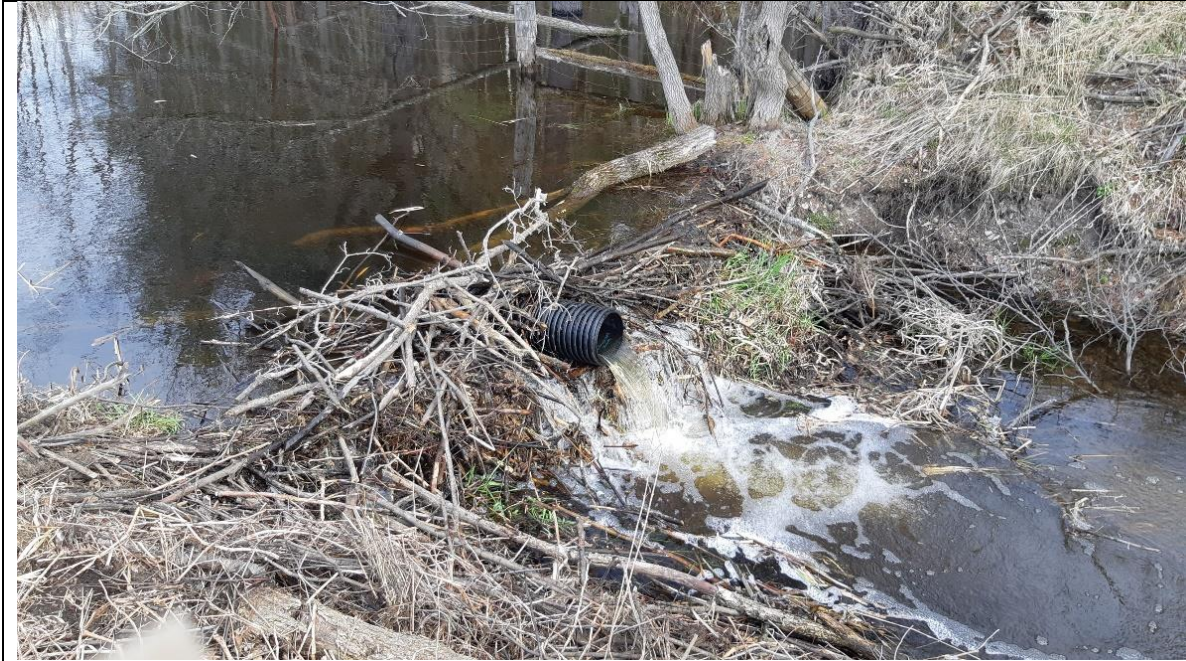
Photo 39: Water flow out of the pipe on initial set-up.
