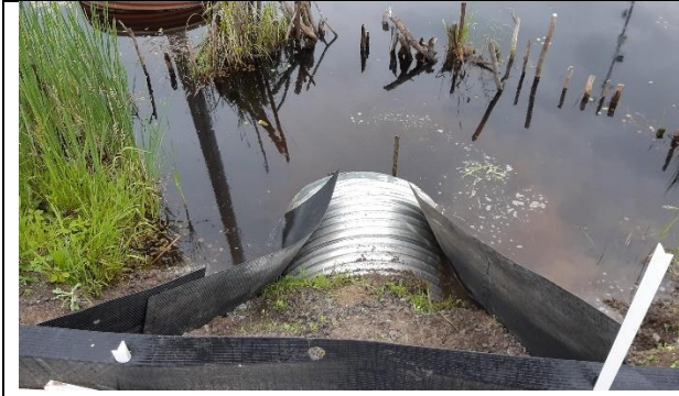
Photo 43: Guide-wall fencing extending from fence to north main culvert entrance on 13-Jun-19.
