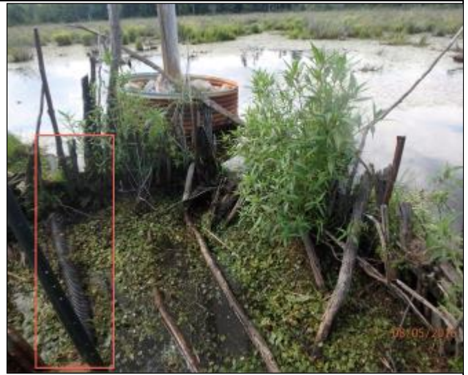
Photo 16: The pipe extended outwards, passing through diversionary dam on west side of culvert, extended westwards, parallel to highway.
