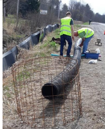
Photo 36: 6-foot 250 mm HDPE Pipe transported and assembled into protective cage on site.
