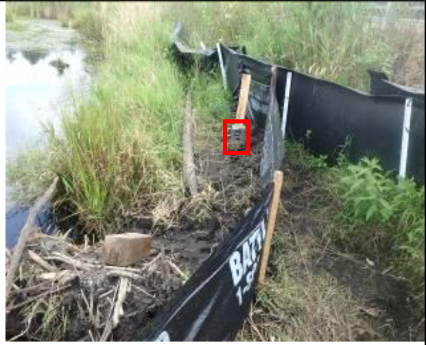
Photo 30: Monitoring camera (red box) set-up on east side of culvert on 12-Aug-2017.
