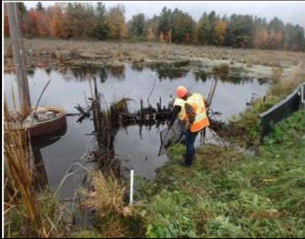
Photo 12: Construction of a diversionary dam around the north culvert entrance on Highway 7
