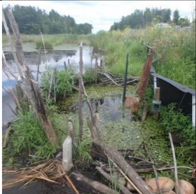
Photo 20: Camera (red box) at west side of culvert facing west side of diversionary dam.
