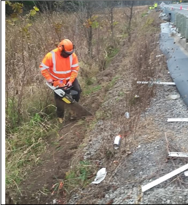
Photo 47: Preparation of ground at road slope for below-grade installation of exclusion fence, 23-Oct-18
