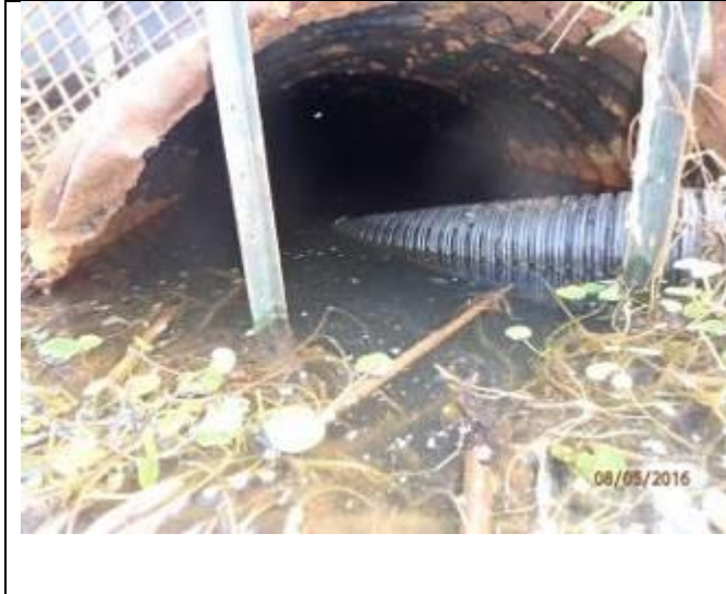
Photo 15: Culvert with two metal t-posts in front of inlet, with pipe anchored on to one (right) post for stability.
