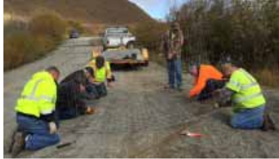
The Oranogan County, WA highway crew builds their first beaver flow device.
