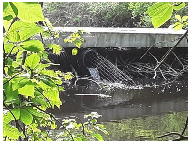
After installation level of pond is reduced one by one foot and maintained by a pipe through the dam
