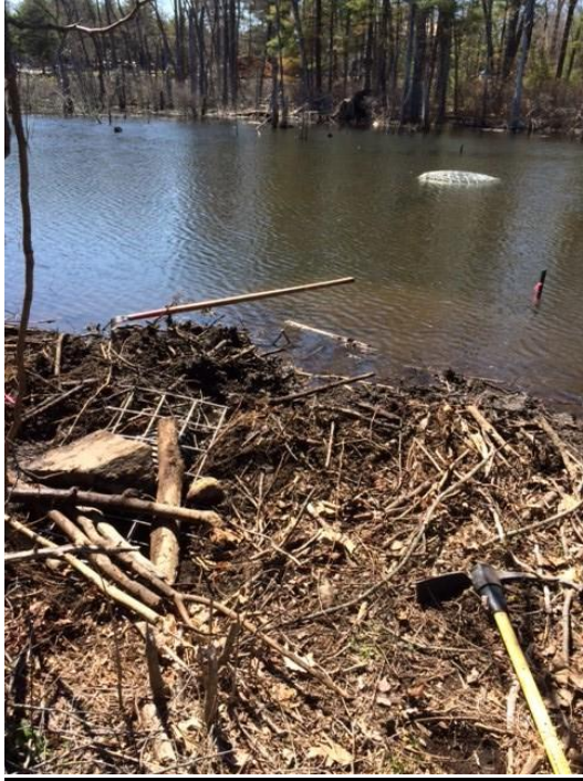
Pond Leveler in Beaver Dam, Rangeway Rd.
